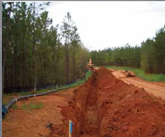
Progress continues as evident with the new roads and utilities being built.
